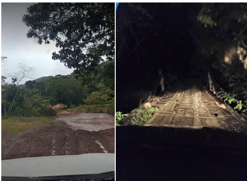
Figure 110. The dirt road and bridges conditions in Acaba Vida settlement.
